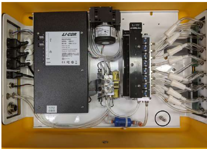
Figure 7-13. The leak test plug is found connected to a post in the lower right side.
