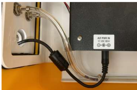
Figure 2-3. Routing the indoor AC to DC power supply through the analyzer connection panel after removing the metal seal.
